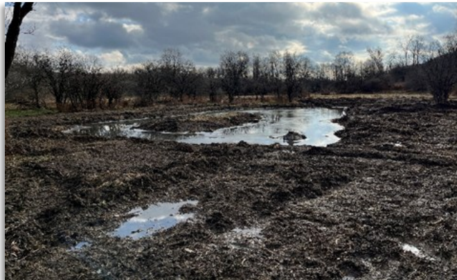
Potholes under construction
