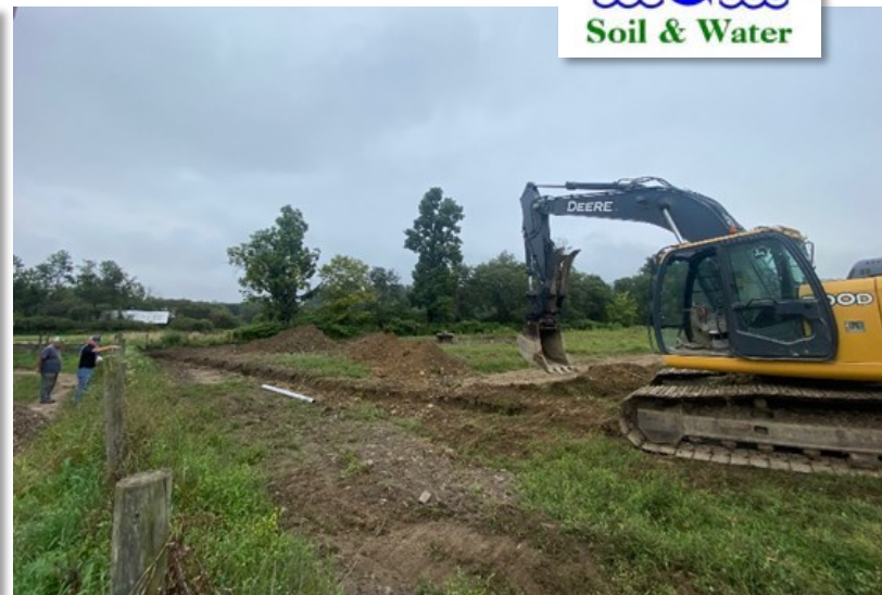
Figure 2. HUA during installation of subsurface drain, photo taken by Broome Co. SWCD staff, September 2024.
