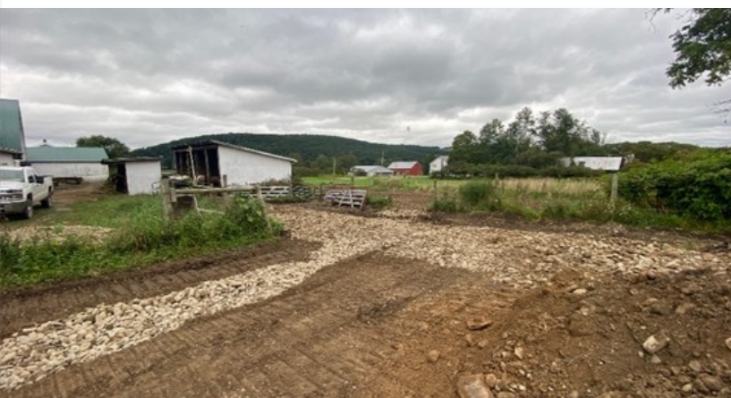
Figure 3. HUA after construction of diversion & subsurface drain, photo taken by Broome Co. SWCD staff, September 2024.
